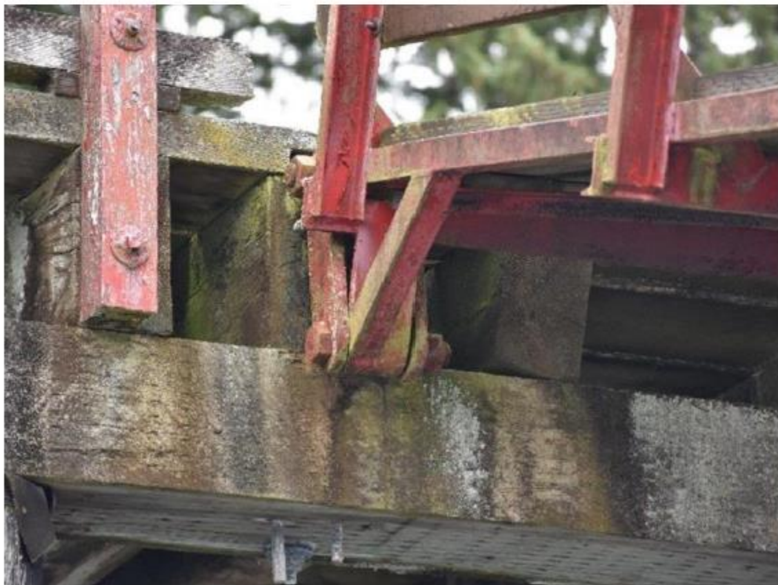
Photo 32 – Gangway Upper Hinge Connection
