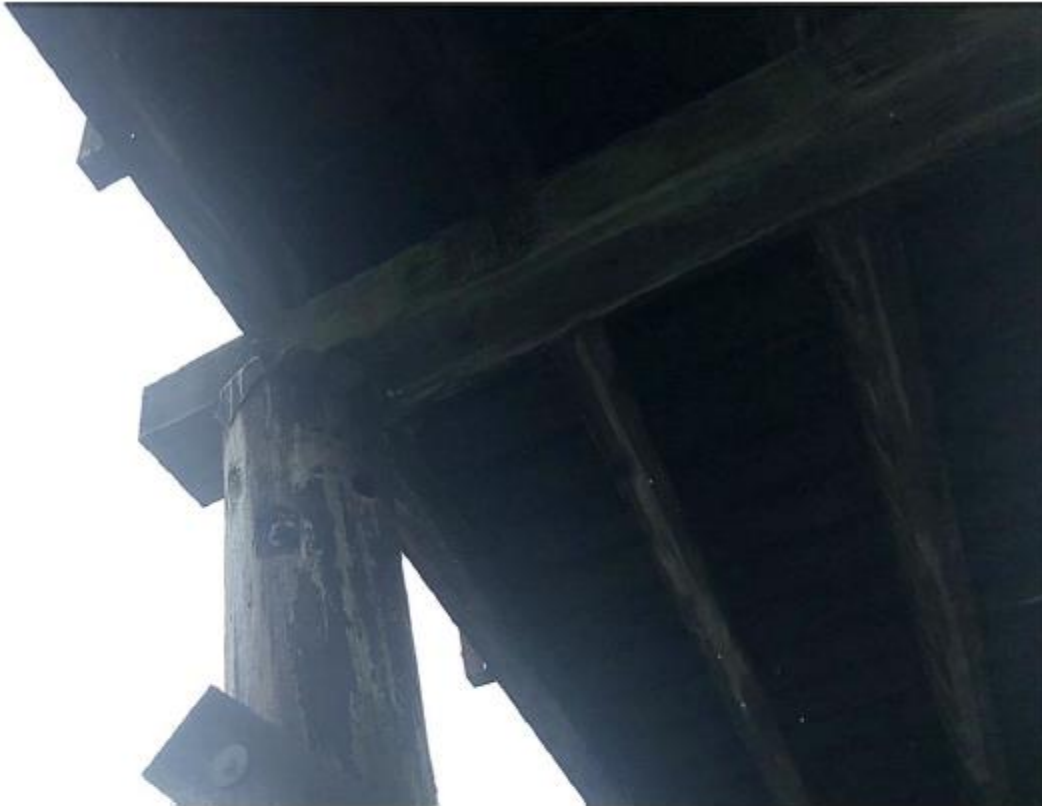
Photo 23 – Hole in Pile 12A
