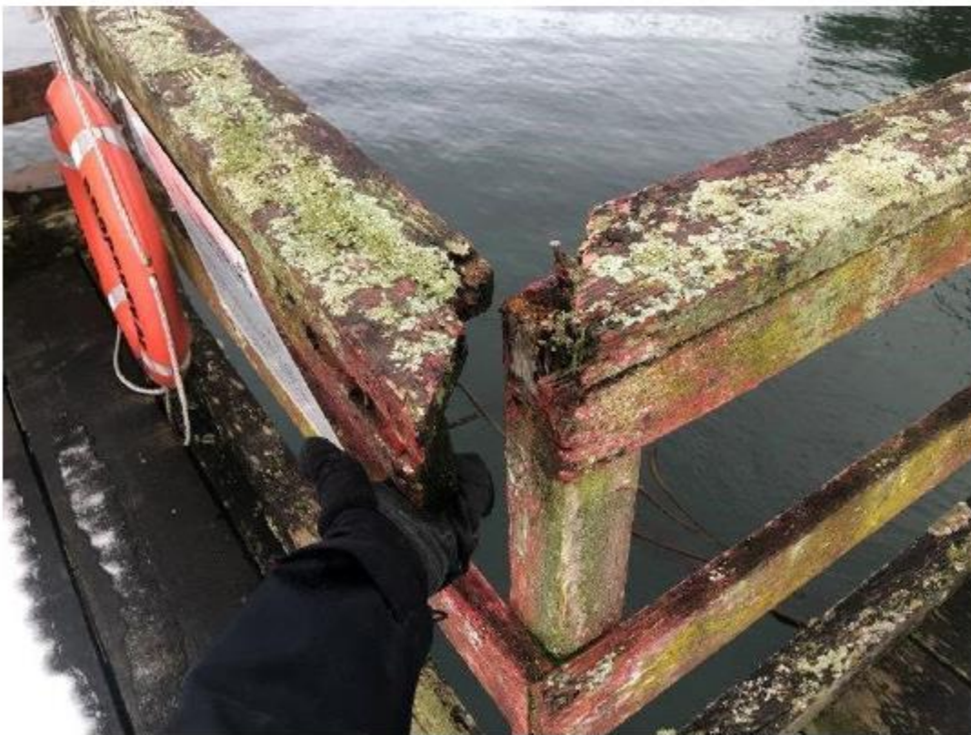
Photo 10 – Handrail deterioration between piles 14B and 14C
