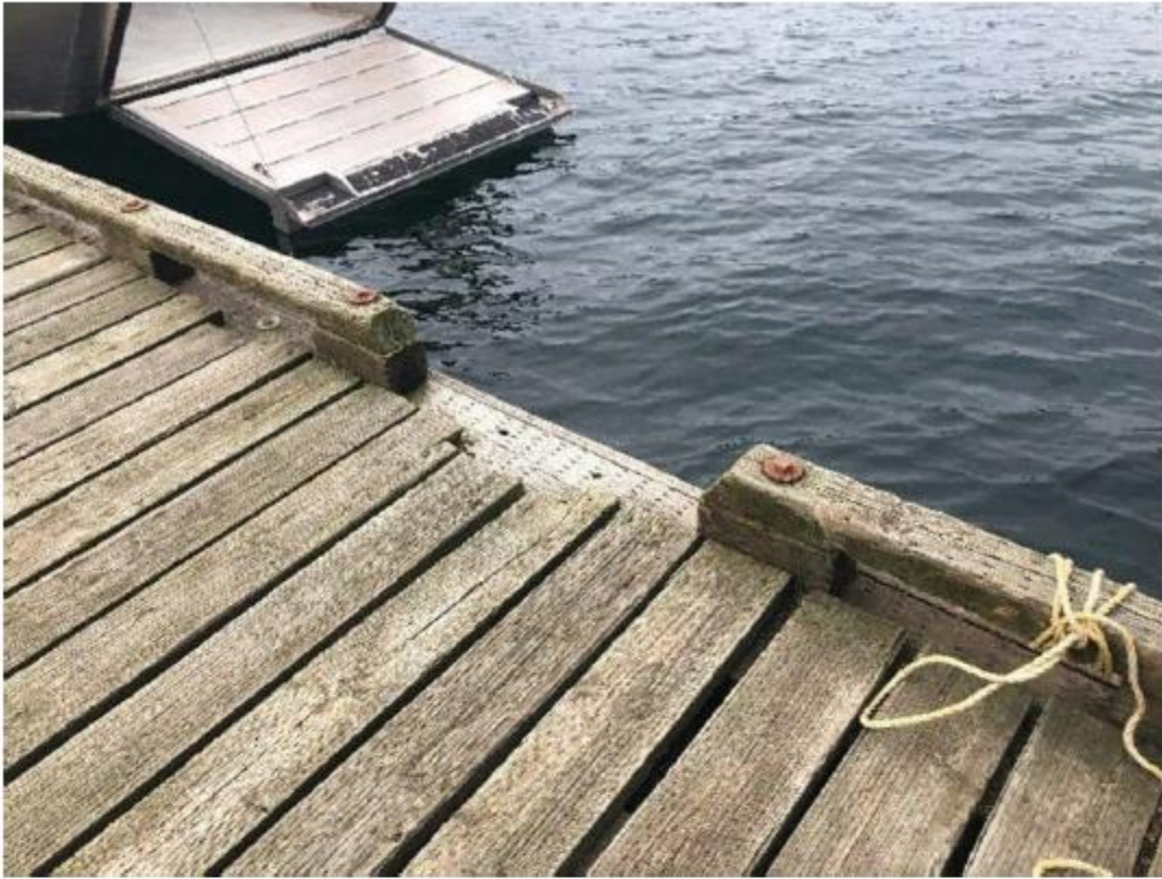
Photo 39 – Missing Bull rail on Float A
