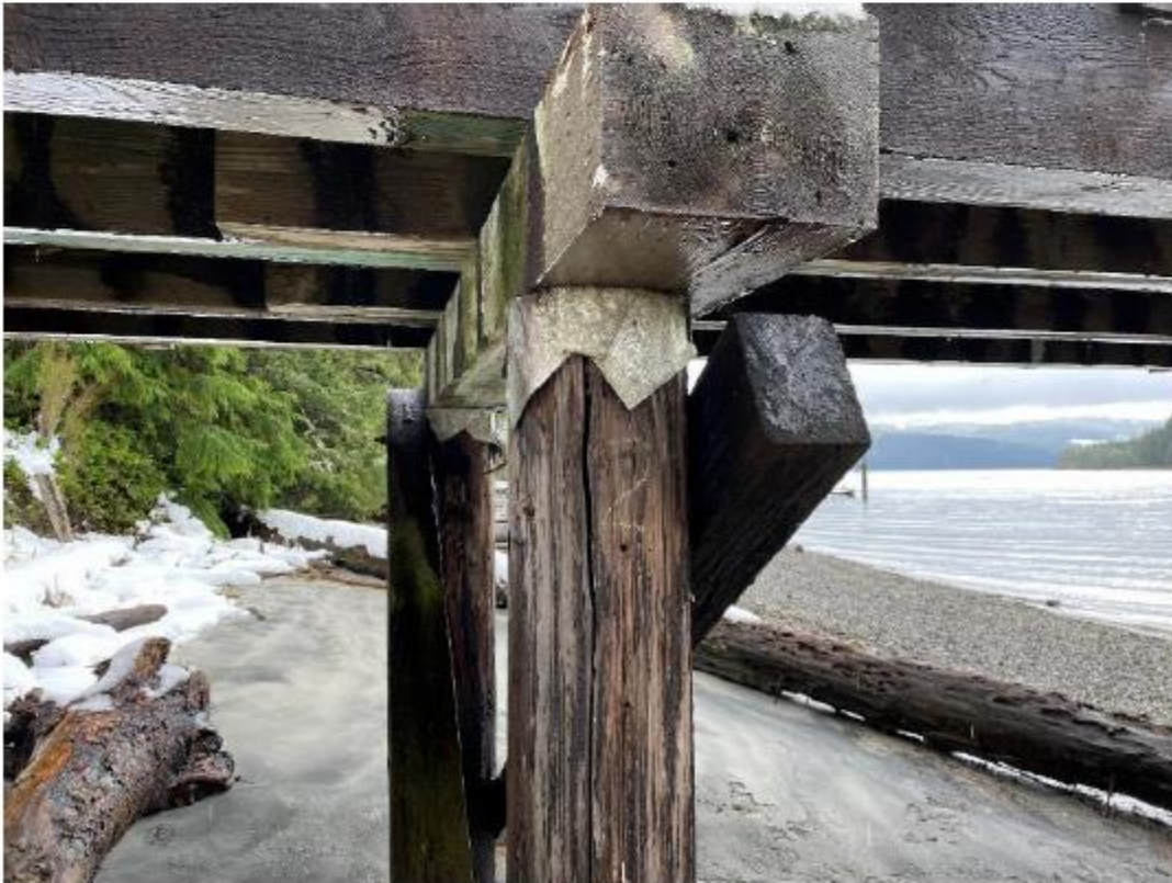
Photo 16 – Split in Pile 3B
