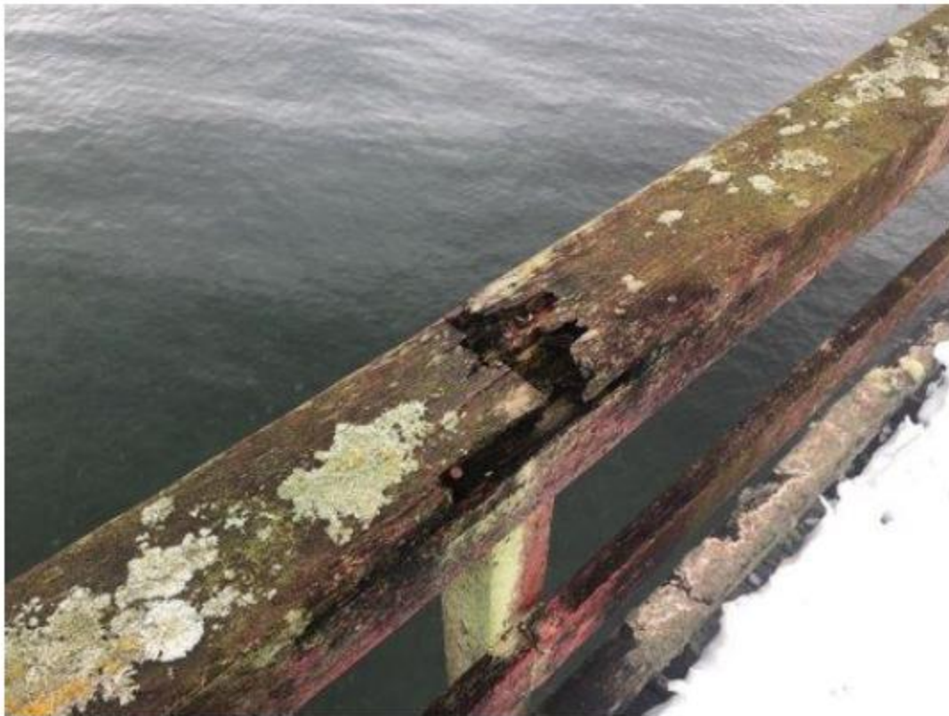
Photo 8 – Handrail deterioration between piles 11A and 12A
