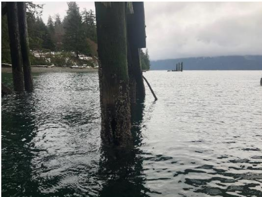
Photo 28 – Fender Pile 15C
