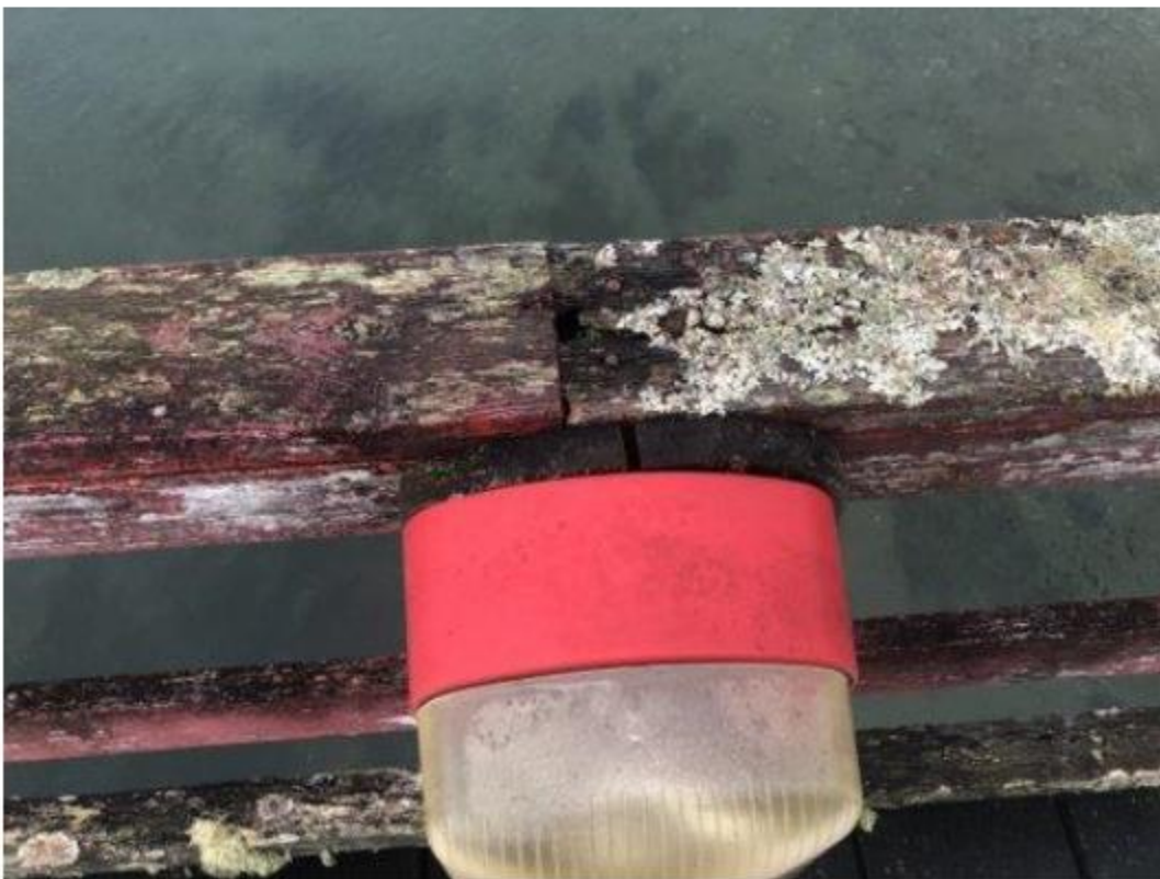
Photo 6 – Handrail deterioration between piles 8B and 9B
