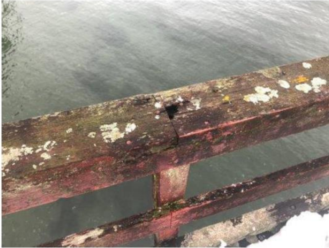
Photo 7 – Handrail deterioration between piles 9A and 10A
