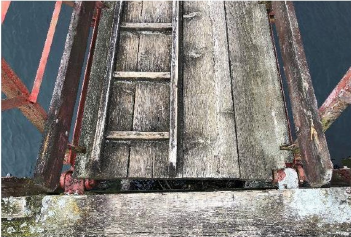
Photo 31 – Gangway Upper Hinge Connection
