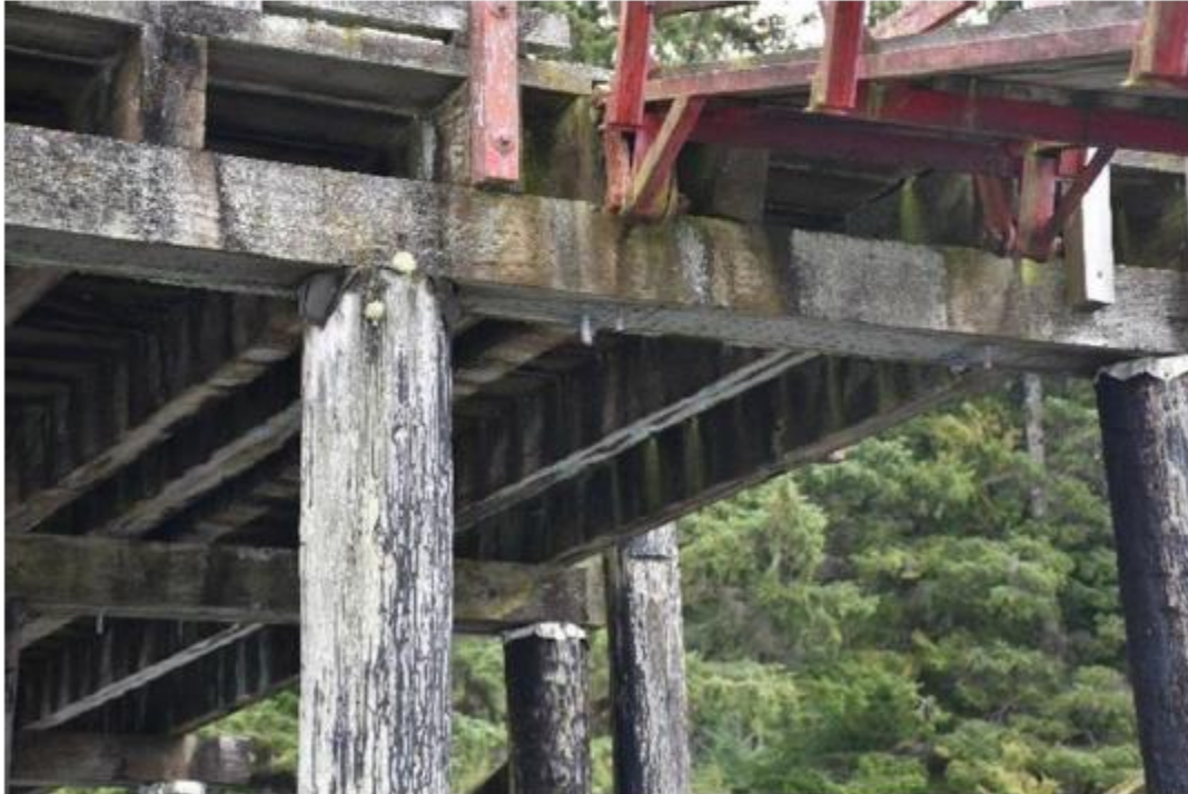
Photo 24 – Moss growth in Pile 15B
