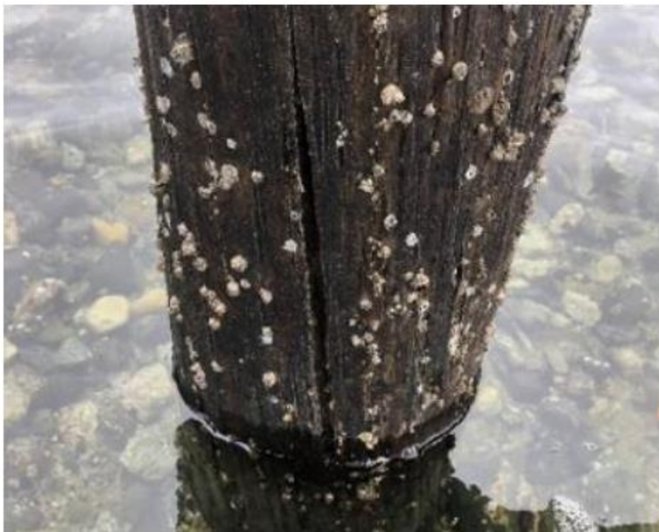
Photo 18 – Split in Pile 5A
