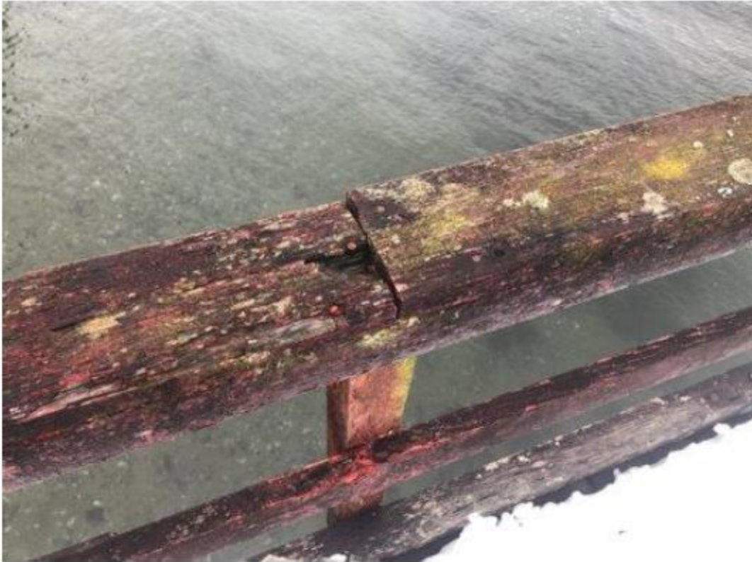
Photo 5 – Handrail deterioration between piles 7A and 8A
