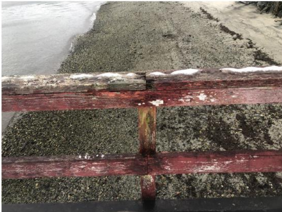
Photo 4 – Handrail deterioration between piles 4B and 5B
