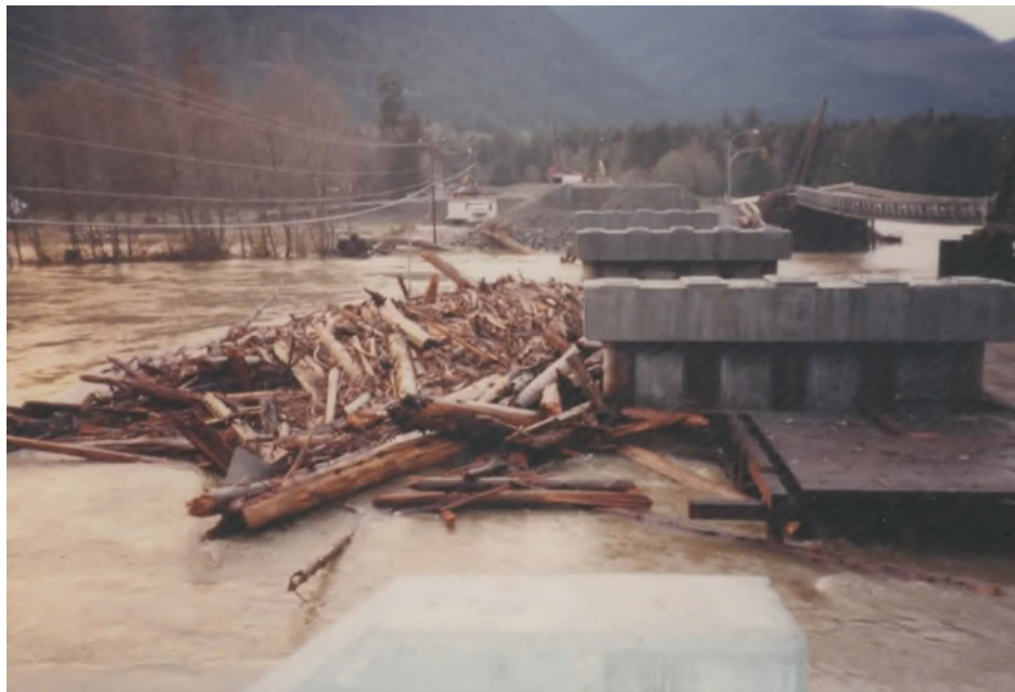
Figure 12: Debris Jam During 1990 Construction of the Sayward Road Bridge Near Sayward
